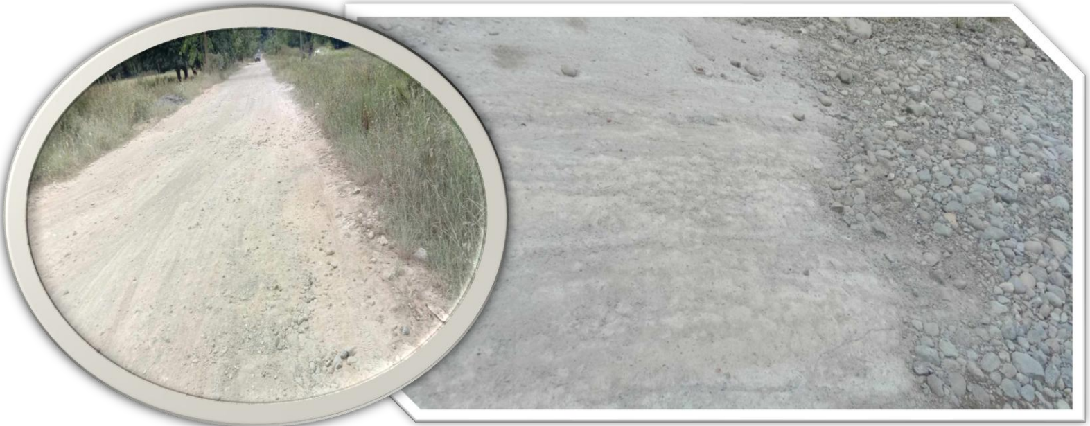
Coal Ash spotted at Bgy. Batang-Batang, Narra, Palawan, along interior roads going to the barangay hall of Batang-Batang
